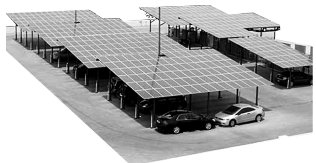
Parking lot covered with solar panels
