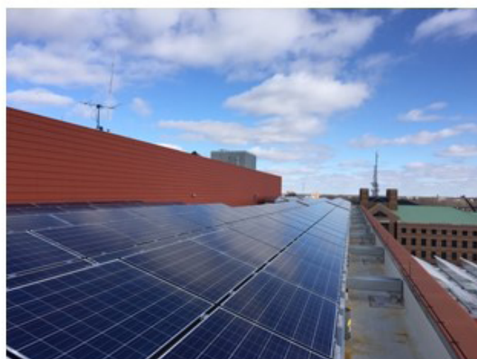
A few of the solar panels mounted on the campus's Electrical and Computer Engineering building 3
