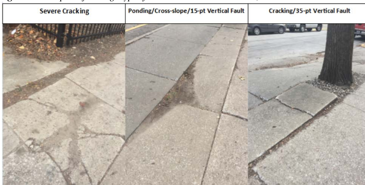
Figure 1: Examples of damage types from Mathews Street Urbana, Illinois.
