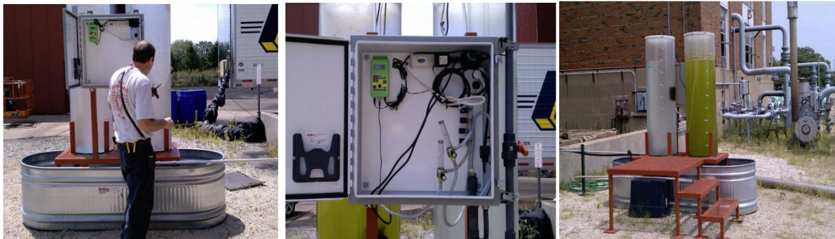
Figure 13. The installation of the weatherized electrical and gas control system was finalized over the summer of 2010 (left & center). The bioreactors were operated over a preliminary trial run (right) to certify its safety for disposal.
