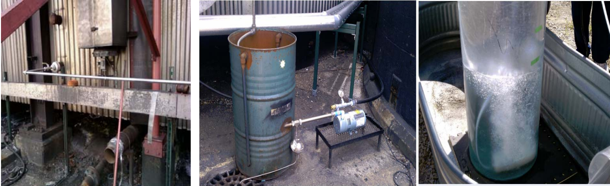
Figure 12. The gas sample line taps into the coal-boiler exhaust stack (left) and is cooled to ambient temperature (middle) before being delivered to the modular bioreactors (right).
