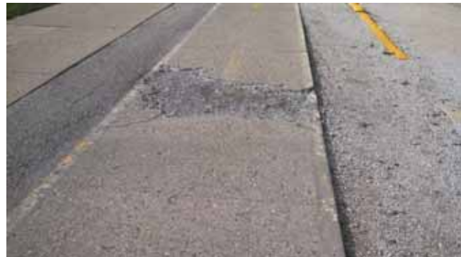
Deteriorated bike path near Burnsides Research Laboratory north of Pennsylvania Avenue. Photo by Geoff Merritt
