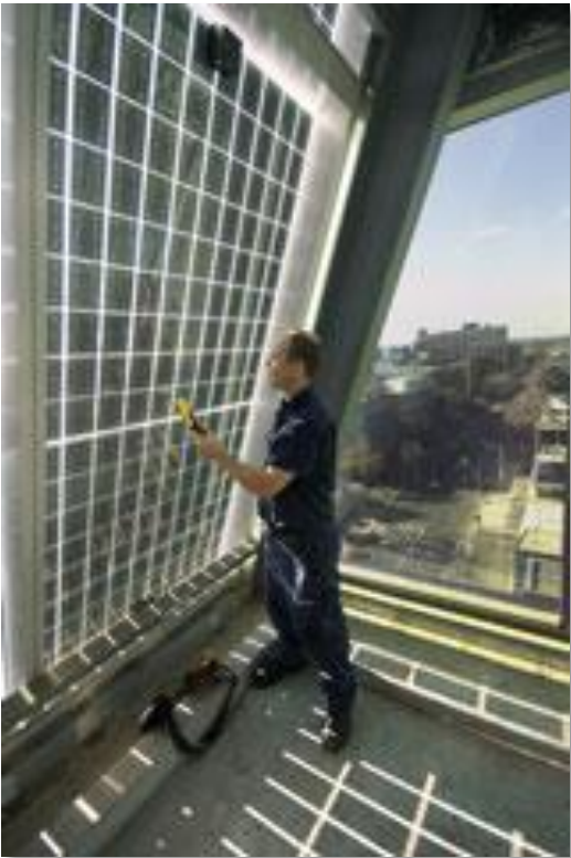
SOLAR ARRAY AT THE ALAN GILBERT BUILDING ON GRATTAN STREET, PARKVILLE.
