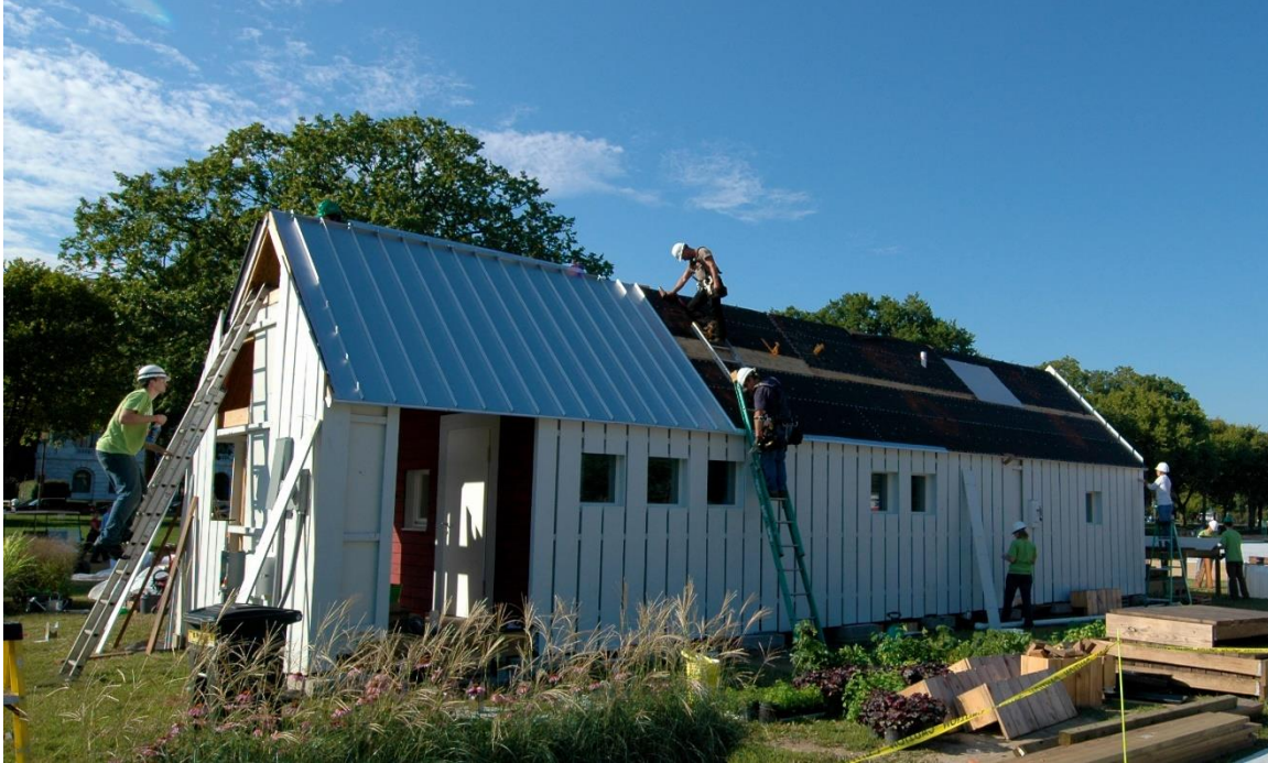
Figure 4. The Gable Home being set up from competition in Washington, D.C., in 2009
