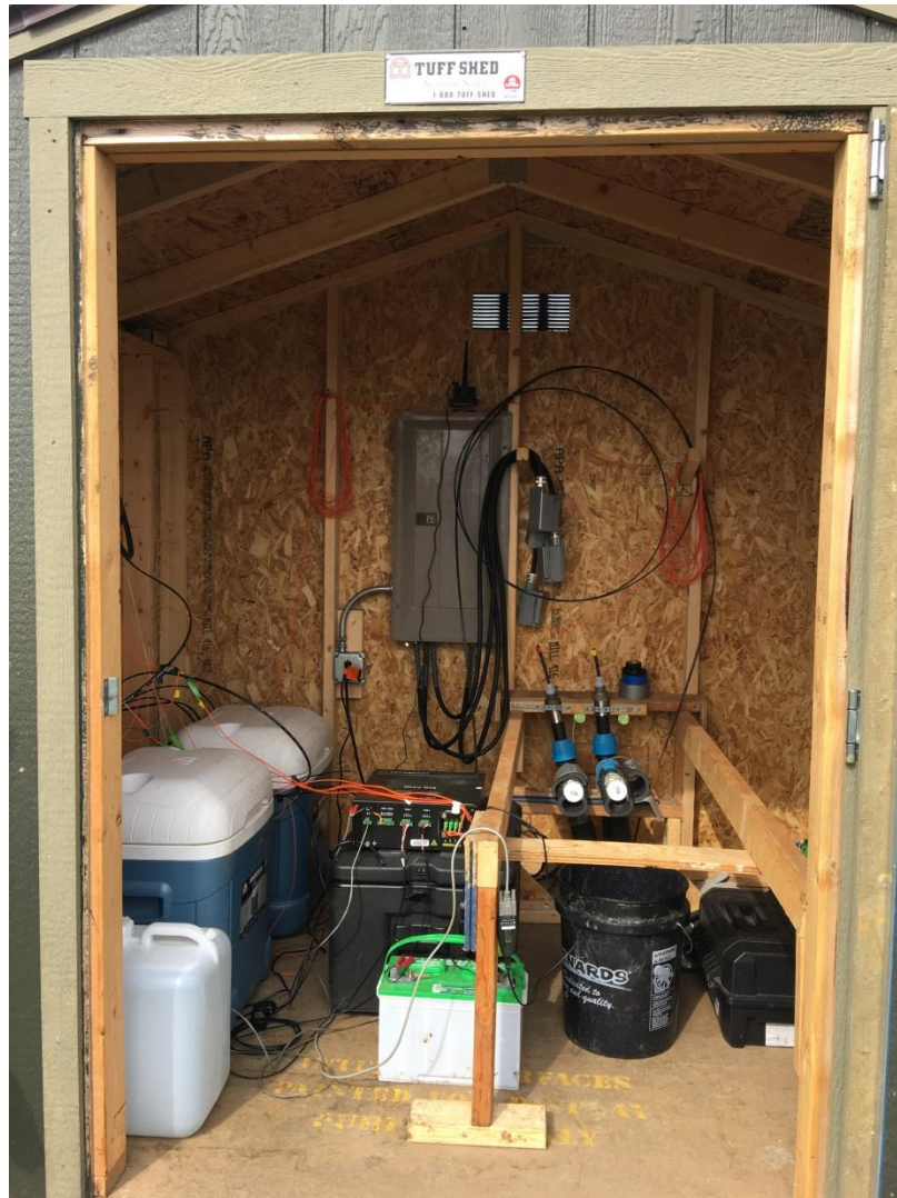
Figure A4. Geothermal test well in Energy Farm
