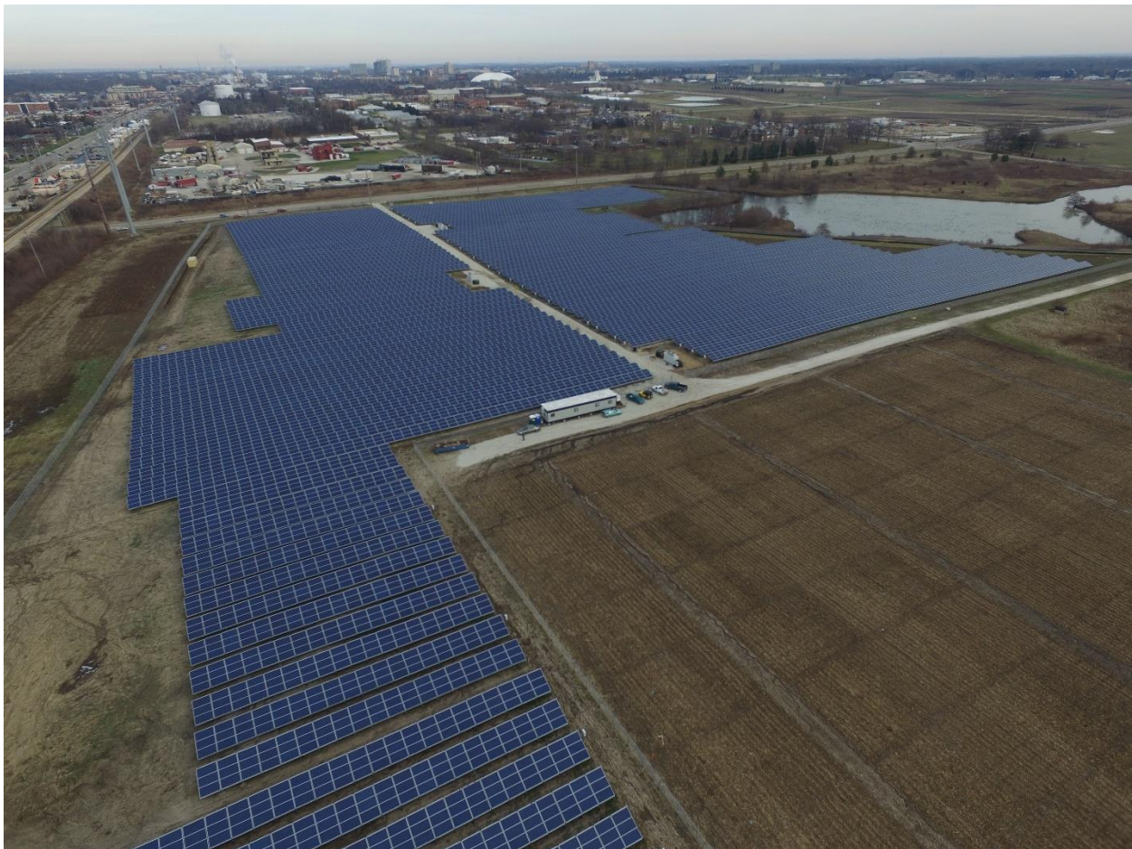
Figure A2. Aerial photo of the Solar Farm (Source: http://www.fs.illinois.edu )
