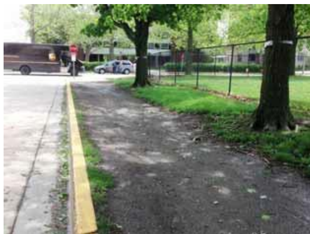
Existing dirt path on the north side of Stadium Drive (#340) Photo by Andy Kopp
