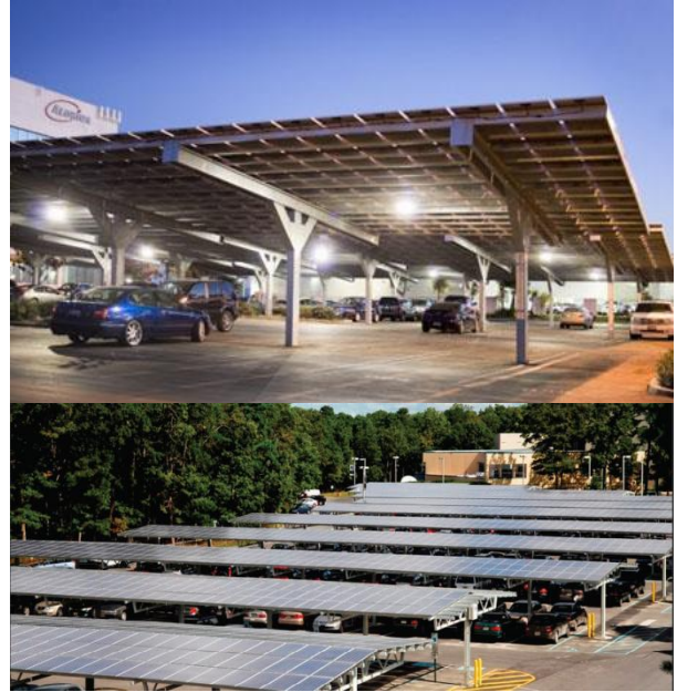
Figure 12. Solar Canopies for Open Parking Lots
