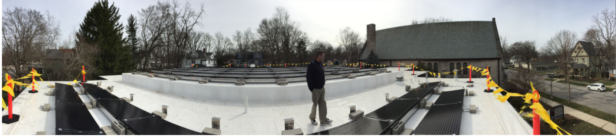
Figure 2: Panoramic view of the final install
