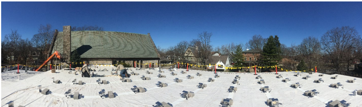
Figure 1: Panoramic view of the solar racking system on the new white roof of UUCUC
