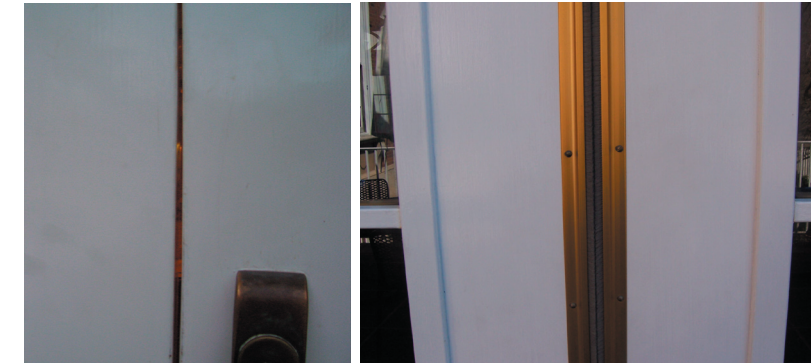
Door with significant gap
